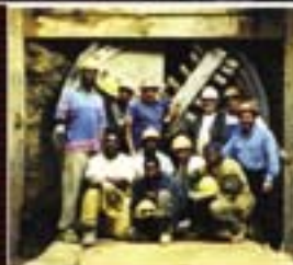
Bottom: Superintendents Jack Jones, J.R. Beachy and crew hole through under the Pentagon. Washington, D.C.
